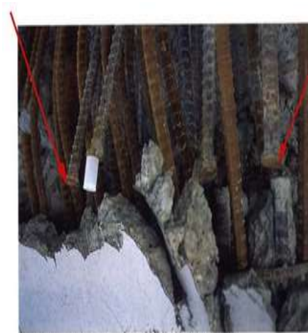
Fig. 6. Failure of "gas-pressure welded" splices in a bridge pier.
